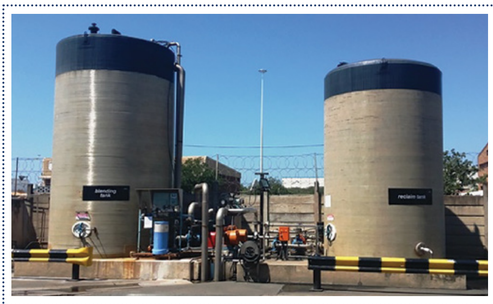
Figure 30. Picture of the recovery and blending tanks.
