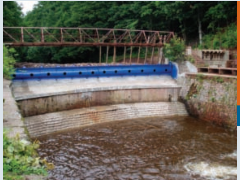
© Olga Kordova, Česká Spořitelna | Weir on the Upa River in Czech Republic, the future site of a small hydro power station. The project is being financed by Česká Spořitelna, a.s. (member of the Erste Group).
