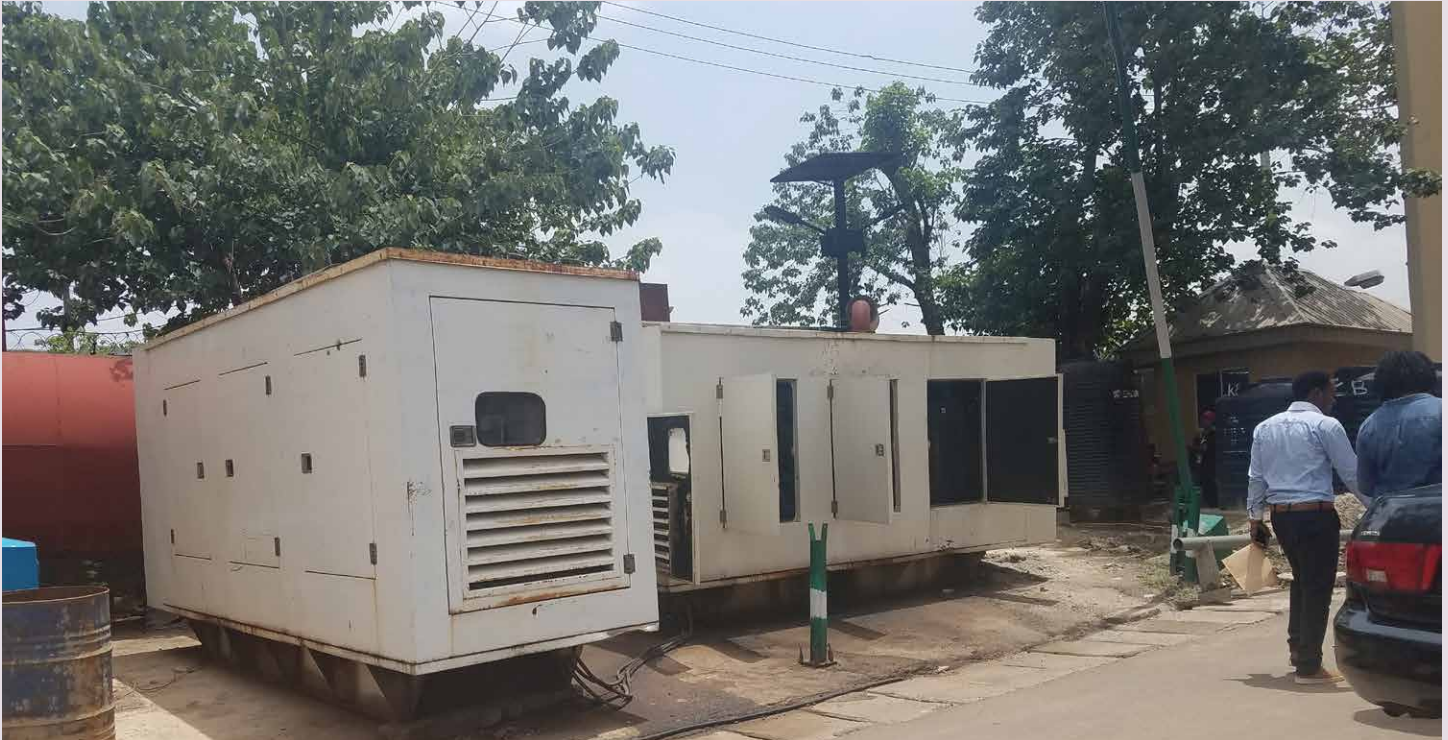
FIGURE 3.4: DIESEL GENERATORS TYPICAL OF THOSE THAT POWER LARGE HOUSING, COMMERCIAL, AND INSTITUTIONAL BUILDINGS
